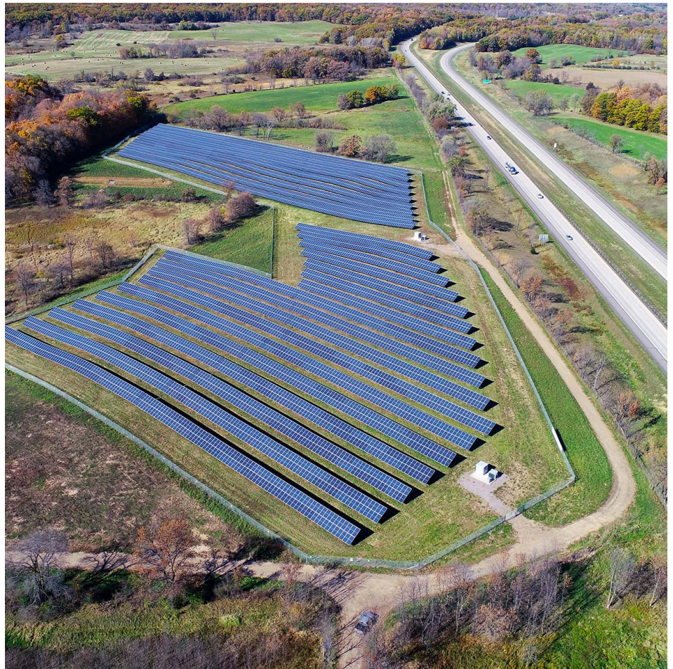
ST. JOSEPH COMMUNITY SOLAR GARDEN, MN | CREDIT: IMPACT POWER SOLUTIONS
