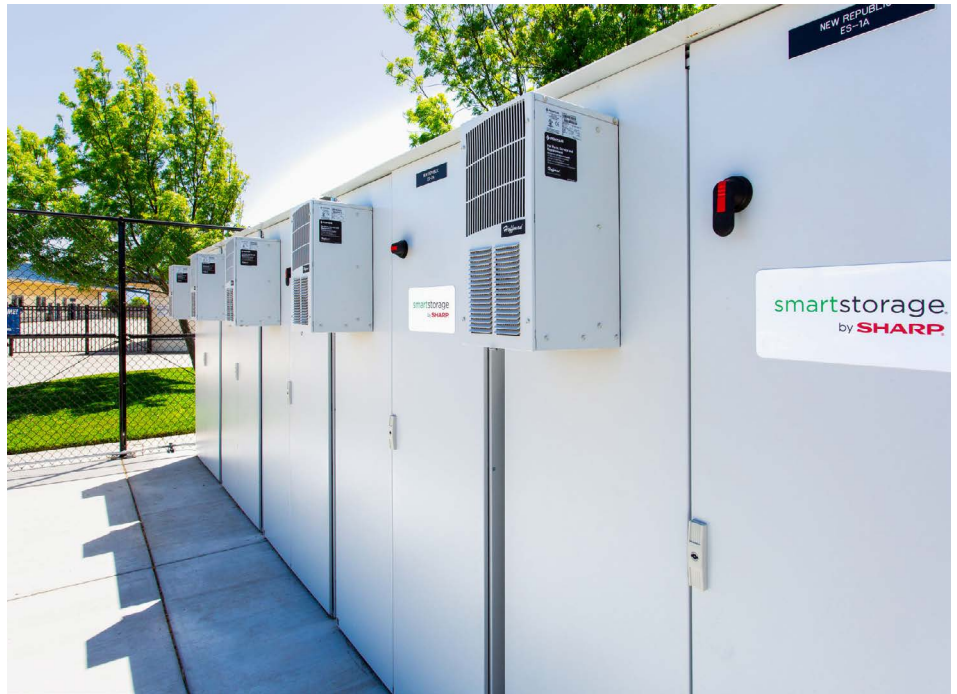
SMART STORAGE SYSTEMS, CALIFORNIA | CREDIT: SHARP
